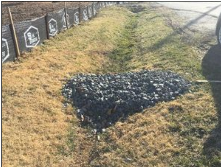
Figure 1. Example Rock Check Dam ( https://stormwater.pca.state.mn.us/index.php?title=Sediment_control_practices_-_Check_dams_(ditch_checks,_ditch_dikes)) )
