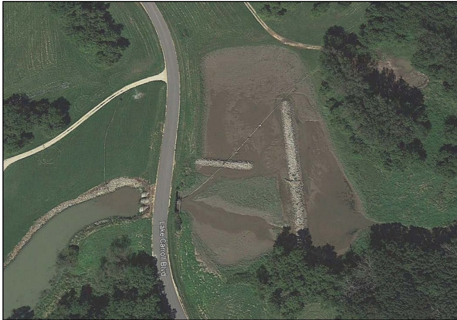
Figure 5. Sediment Basin Located on a Large Lake in Rural NW Illinois – Aerial View
